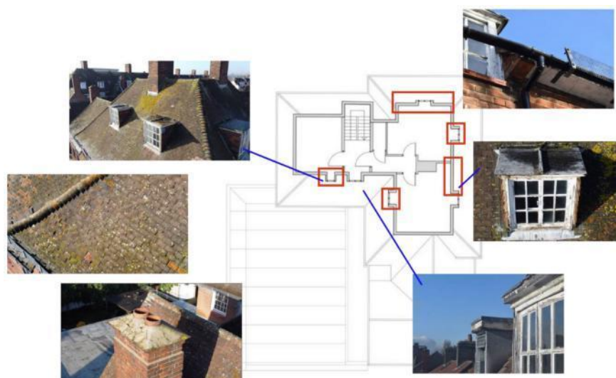
Examples of the building's current state of disrepair.
